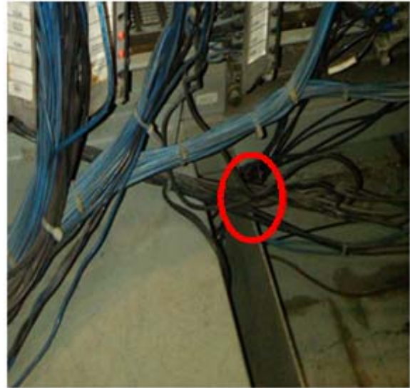
Fig17: Top plate taken aside to see the cables over the vertically mounted support
