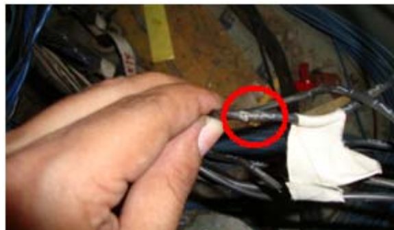
Fig18: Cut on the Grounded Cable
